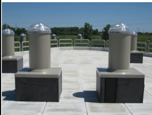
Over 20 photo tubes were installed in the roof to bring natural light into the building interior.
