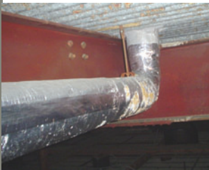
Condensation on ductwork
