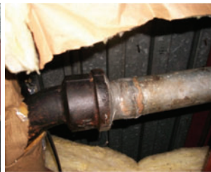
Leaking plumbing pipe below roof drain
